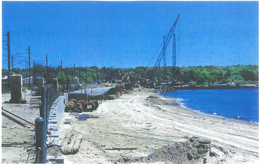
Figure 4. Looking eastward along "The Bar," the concrete sheet pile wall is visible at the left. Cranes are working near the bridge location.
