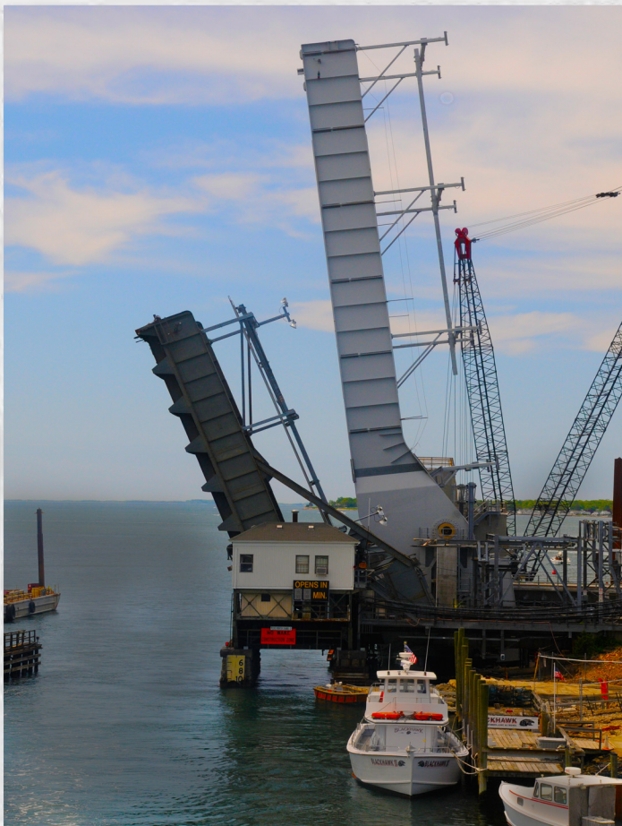
Photo taken on May 20, 2012, from the Route 156 highway bridge. The 1907 span is 45' long and the new span is 138' long.
