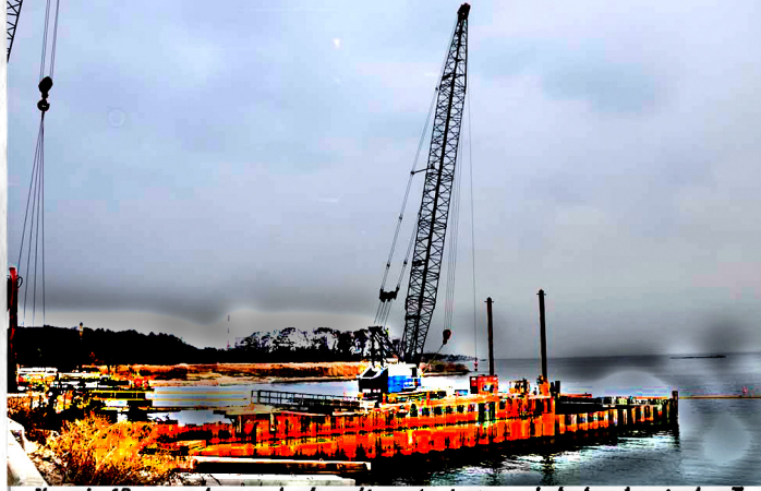
November 16: a crane places sand and gravel to create a temporary dock where dump trucks will receive materials from barges for the Overlook project. - photo by R.S. DeSanto
